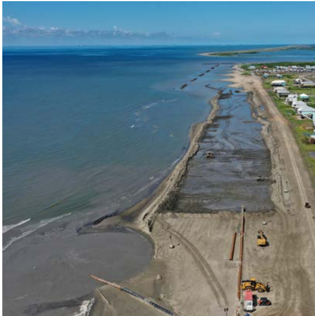
Top: Segmented Breakwaters protect the west end of Grand Isle Middle: Beach nourishment activities on the Grand Isle shoreline
