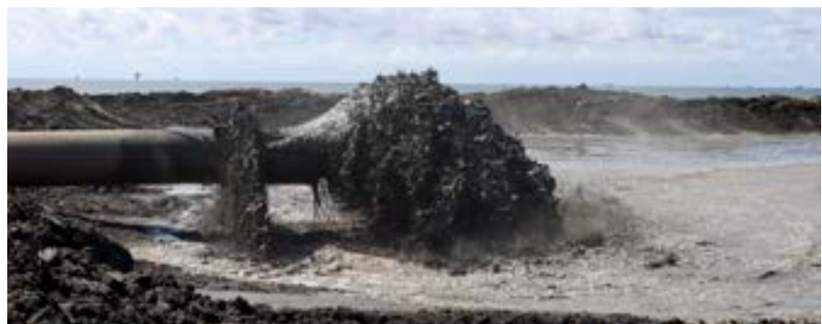
Dredge pipes pump material from the Gulf of Mexico to Grand Isle beach
